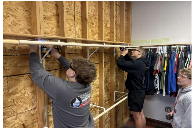
Construction Technology students assist with installing new shelving in the school sponsored Caring Closet
